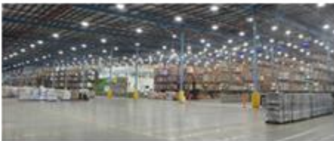
Smart LED Highbay Lighting
